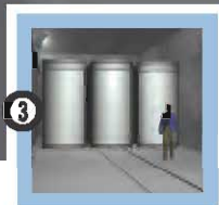
Resin Liner Shields within ILW Vault
