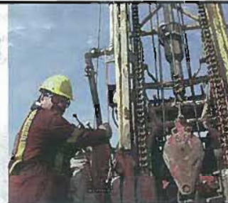
Davidson driller Paul Marice drilling one of the six deep boreholes, which is part of the geoscientific site characterization program to verify the Bruce site as a location for OPG's proposed DGR.
