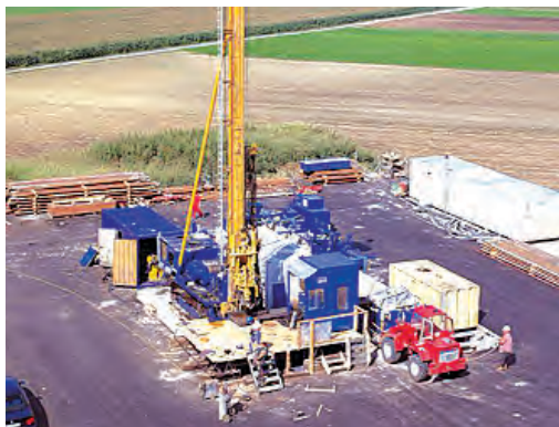
Borehole drilling at the Bruce site, similar to what is portrayed in this photo of Alberta, will be erected on a temporary basis to uncover invaluable information about the suitability of the Bruce site as a host for a long-term storage facility for low and intermediate level nuclear waste.
