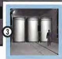
3 Resin Liner Shields within ILW Vault
