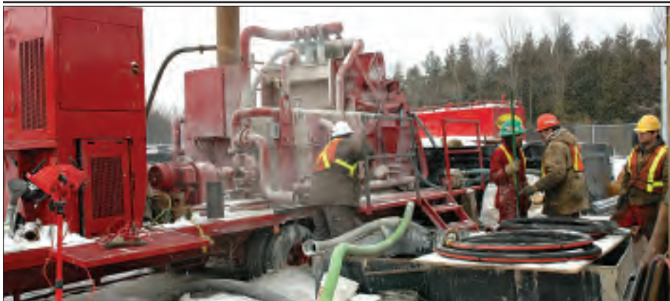
Phase one of the geoscientific site characterization activities for the Deep Geologic Repository have begun at the Bruce site. Drilling and coring of the first bore hole, which will go down to 450 metres is currently underway. The silt shaker removes particles from drilling fluid used in the process.
