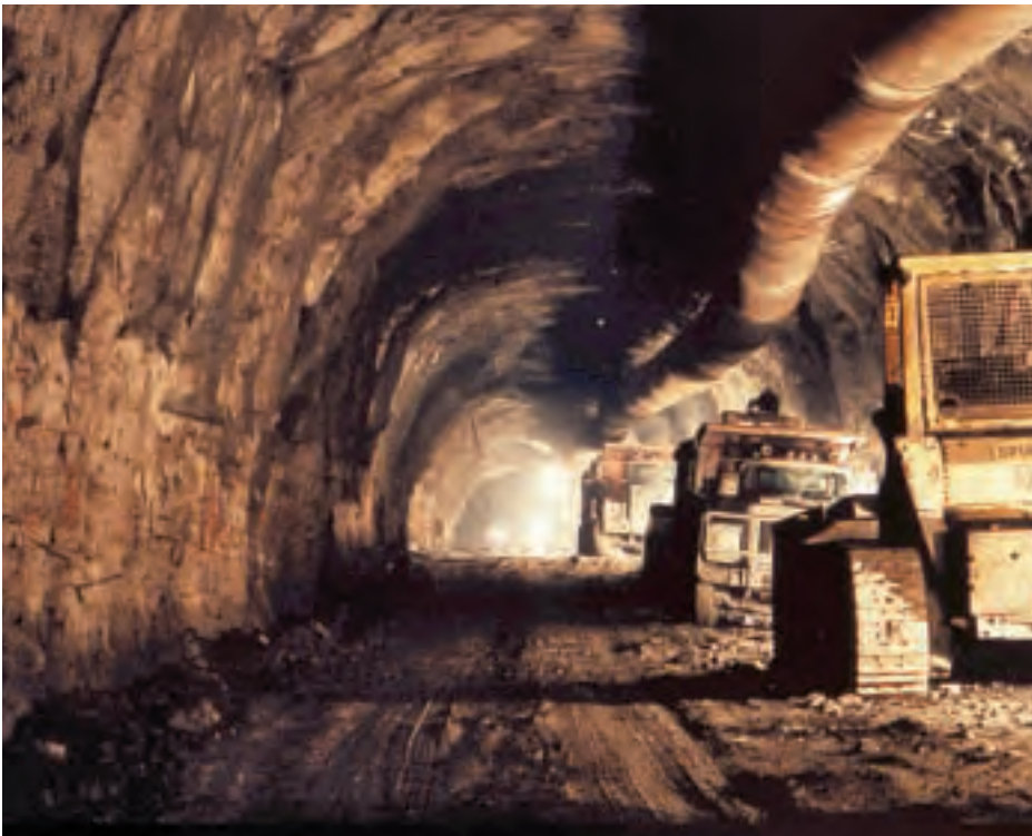
Construction of the cooling water intake tunnel at Darlington in the Cobourg Formation provided evidence that the formation can sustain a stable, dry opening.
